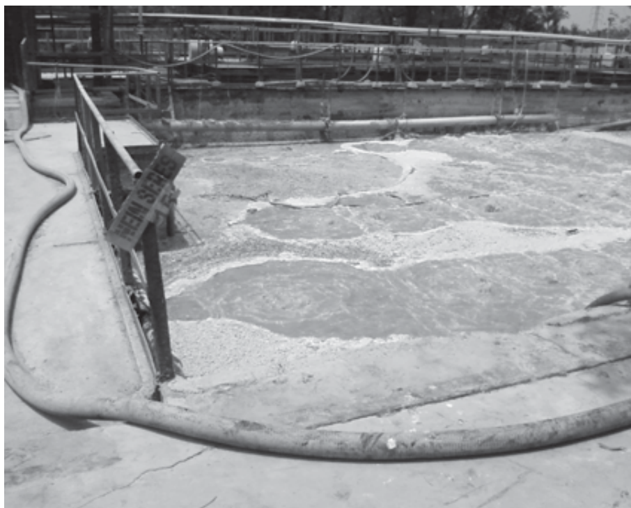
Effluent water being treated in the company
