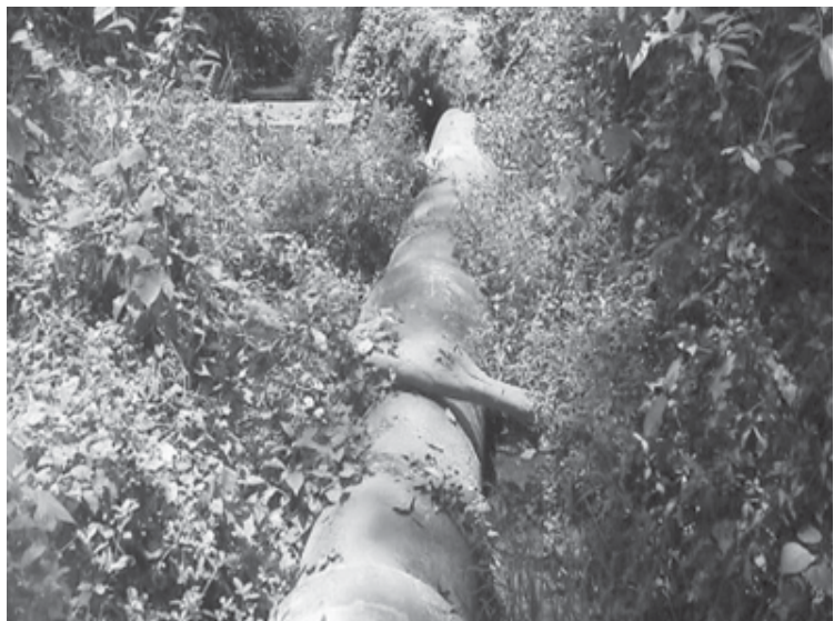
Huge concrete pipe carrying effluents to Chalakkudy River
