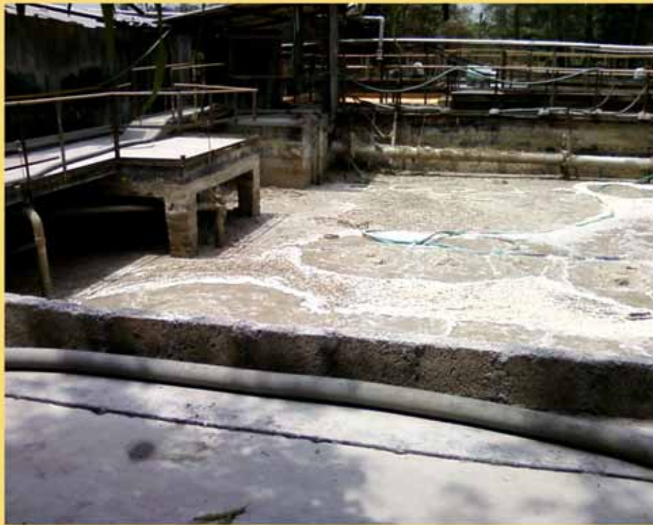
Fig. 10 : Effluents being treated
